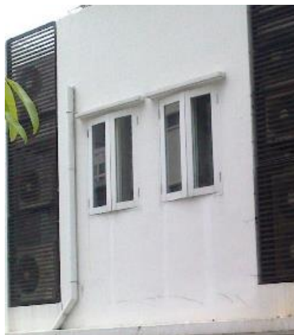
A/C ledges: Louvers with insufficient depth
