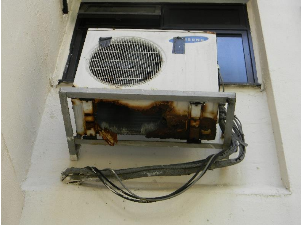
Figure 5: Badly corroded bracket
